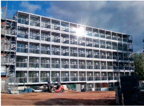
When completed in time for semester one 2010, the six-storey building will include a mix of apartments for couples and singles, as well as a common room, laundry and bike storage.
