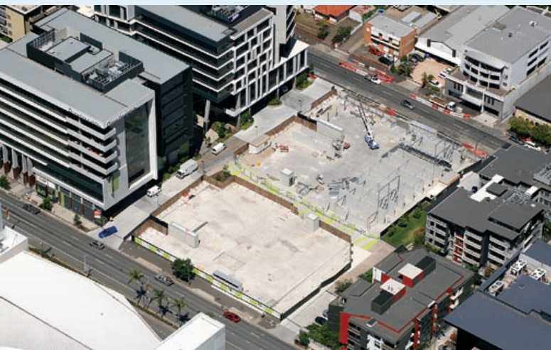
Under construction is Terrace Row SW1 in South Brisbane – inspired by London's 19th century townhouses in that city's own SW1.
